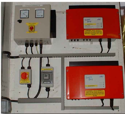
*Above, an installation showing 2off SWR2500 (windy Boy) inverters mounted with a Proven ECM controller, isolator switch and DC disconnect.
